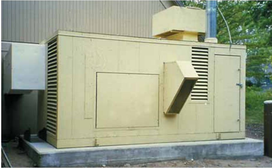
The DESI-AIR natural gas desiccant system / heating unit controls moisture to extend months of operation and increase revenue for Blake Ice Arena.
